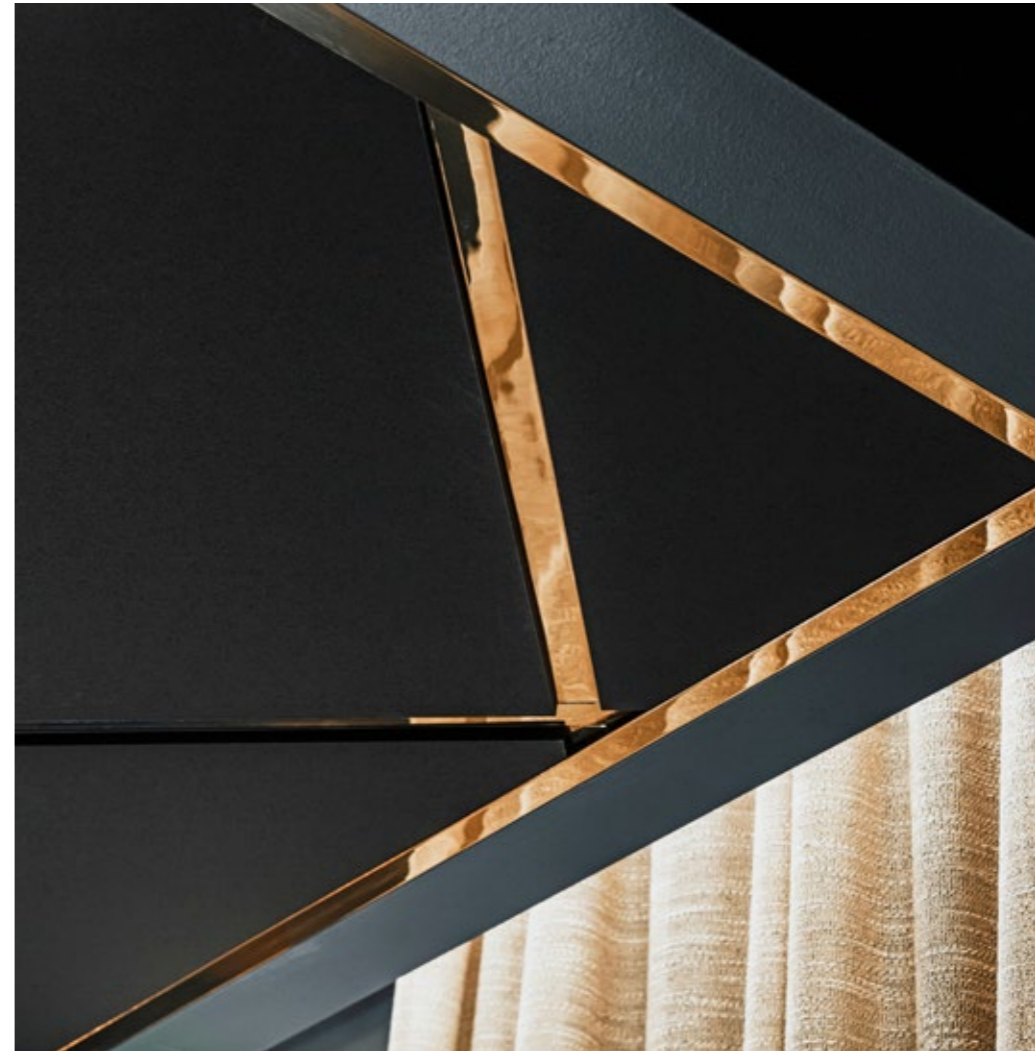
At Jacy'z, Ecophon Focus™ has played an important role in extending the design concept to the ceiling through the choice of colour and unconventional installation. Looking at design and acoustics from every conceivable angle.
